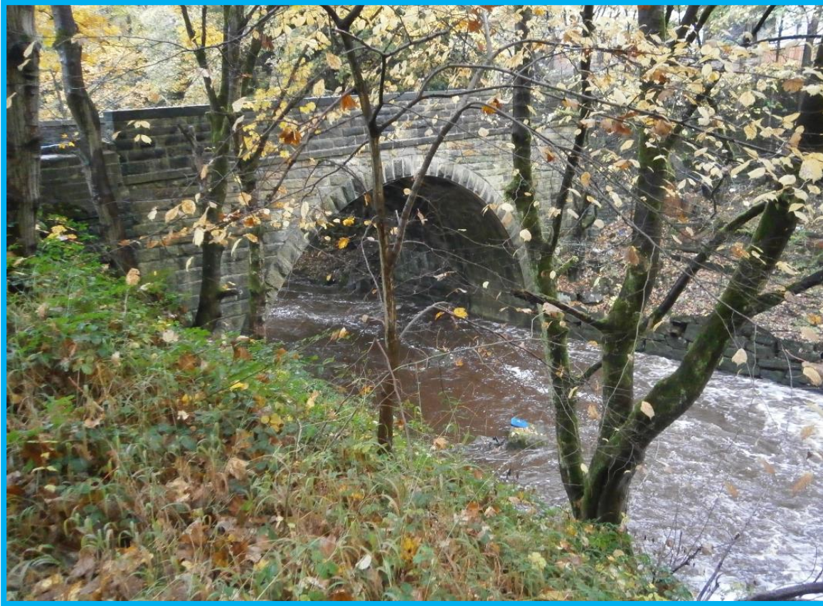
Fig 30 View of substantial River Colne bridge supporting Low Westwood Road (Bargate Bridge), downstream of weir.
