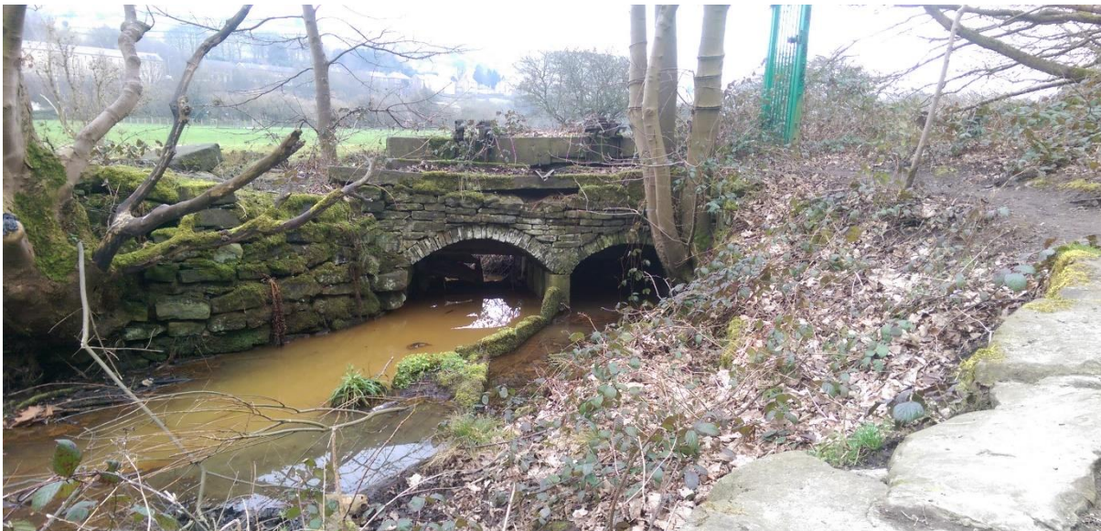
Figure 12 –Looking upstream, offtake sluice from the River Colne to the mill channel
